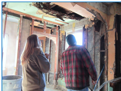
Melody Picciotti and Mike Cendrowski examine the demolition work for their future home.
